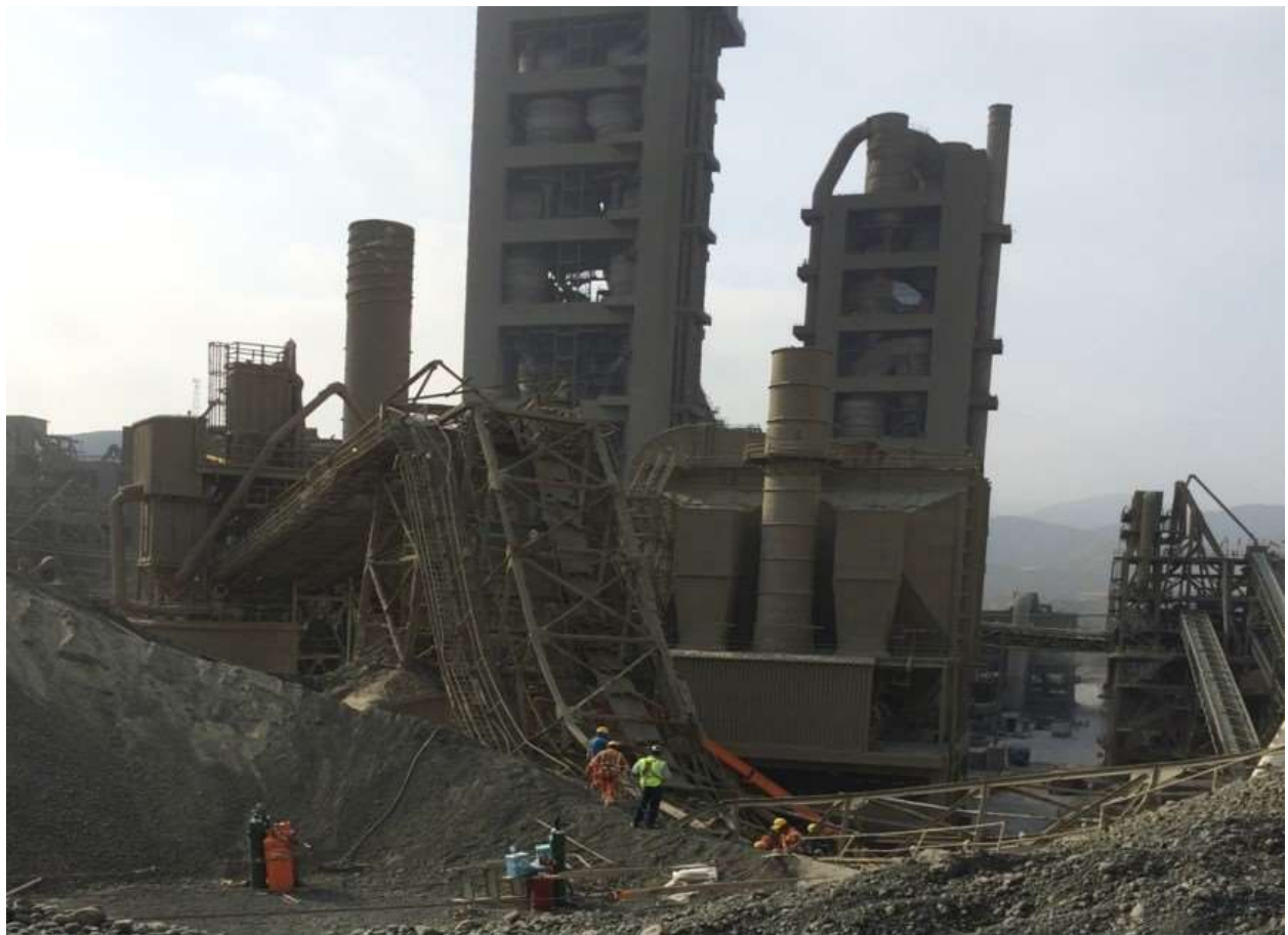
INVESTIGATION OF THE COLLAPSE OF THE METALLIC STRUCTURE OF A CONVEYOR LINE
