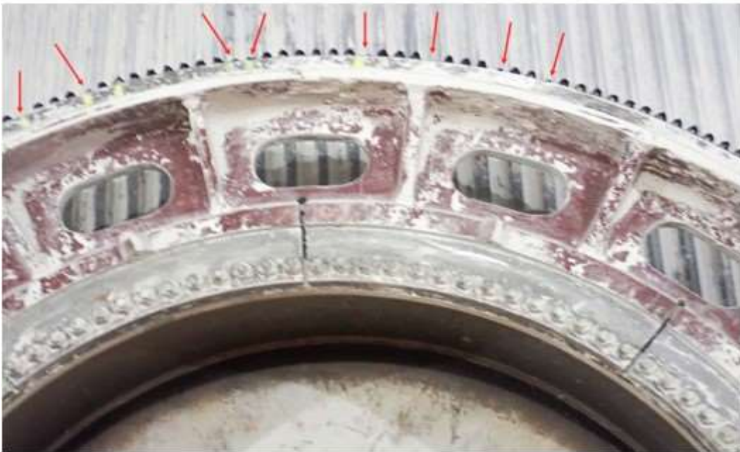
FAILURE OF A MILL RING GEAR IN A CEMENT PLANT
